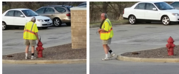
Figure 4. Nearly 100 days ago, listening for water leaks with acoustic hydrophones and data correlators.
